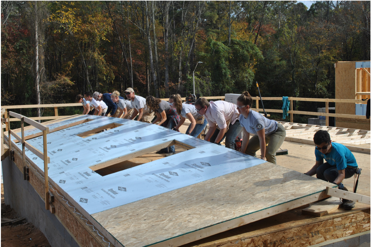
Students at Franklin build character through service. The 11th grade Learning Expedition explores the issue of housing costs and poverty in Asheville, culminating with the Habitat for Humanity Student Home Build.
